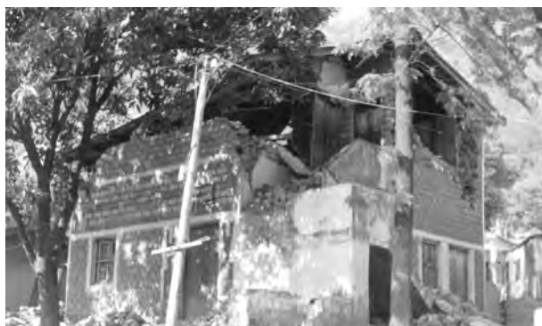
Figure 7.1 : A Damaged Building Due to an Earthquake
