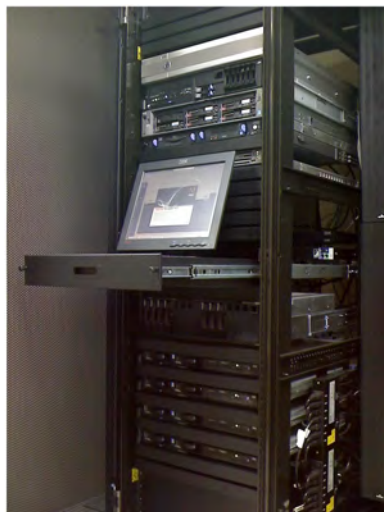
Fig. 4.5 : Rack mounted servers
