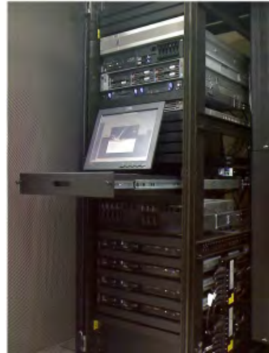
Fig. 4.5 : Rack mounted servers
