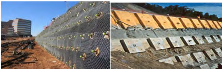
Fig. 8.12 :Rock bolts to prevent slope failure
