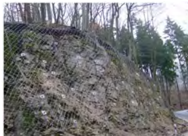
Fig.8.11: A slope covered with wiremesh
