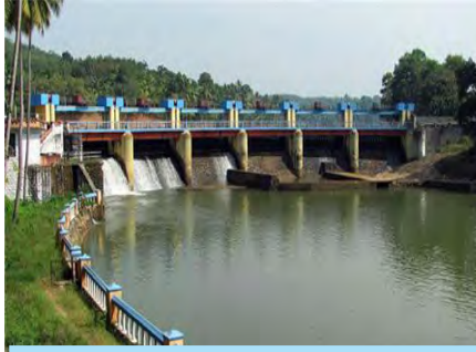
Fig. 8.8 : A flood gate in Aruvikkara-Kerala
