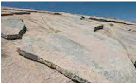
Fig. 4.33: Sheet joint in granite
