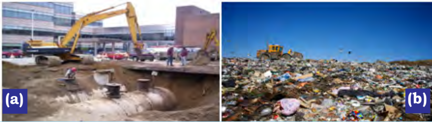
Fig. 6.15 (a) & (b): Storage tanks and landfills as sources of groundwater contamination
