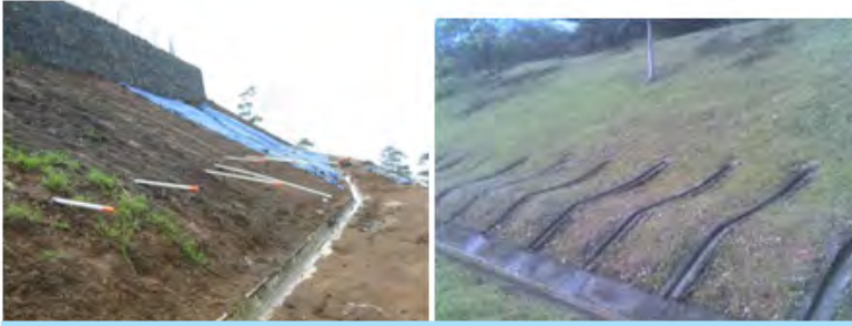
Fig. 8.13: Drainage pipes along slopes.
