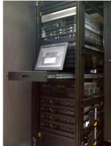
Fig. 4.5 : Rack mounted servers
